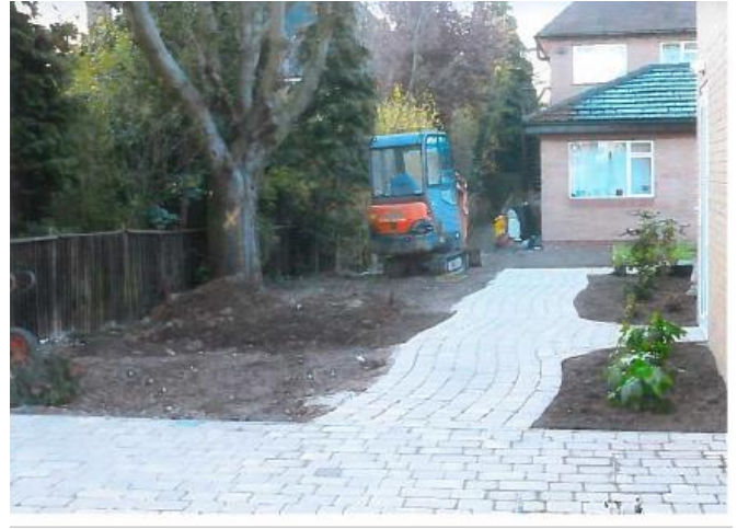
Physical damage and Tree removal
